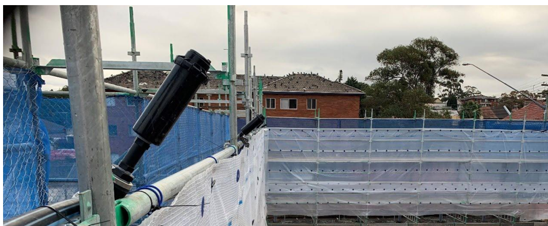
Figure 2: Ring sprinkler system
